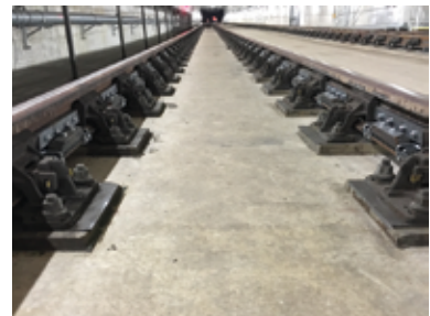
Tuned Dampers on ballastless track
