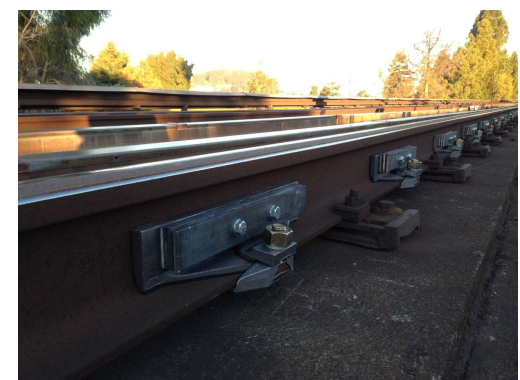
Tuned Dampers on ballastless track
